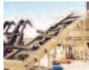
ST-100 Shredder and feed conveyor processing spent military munitions.
